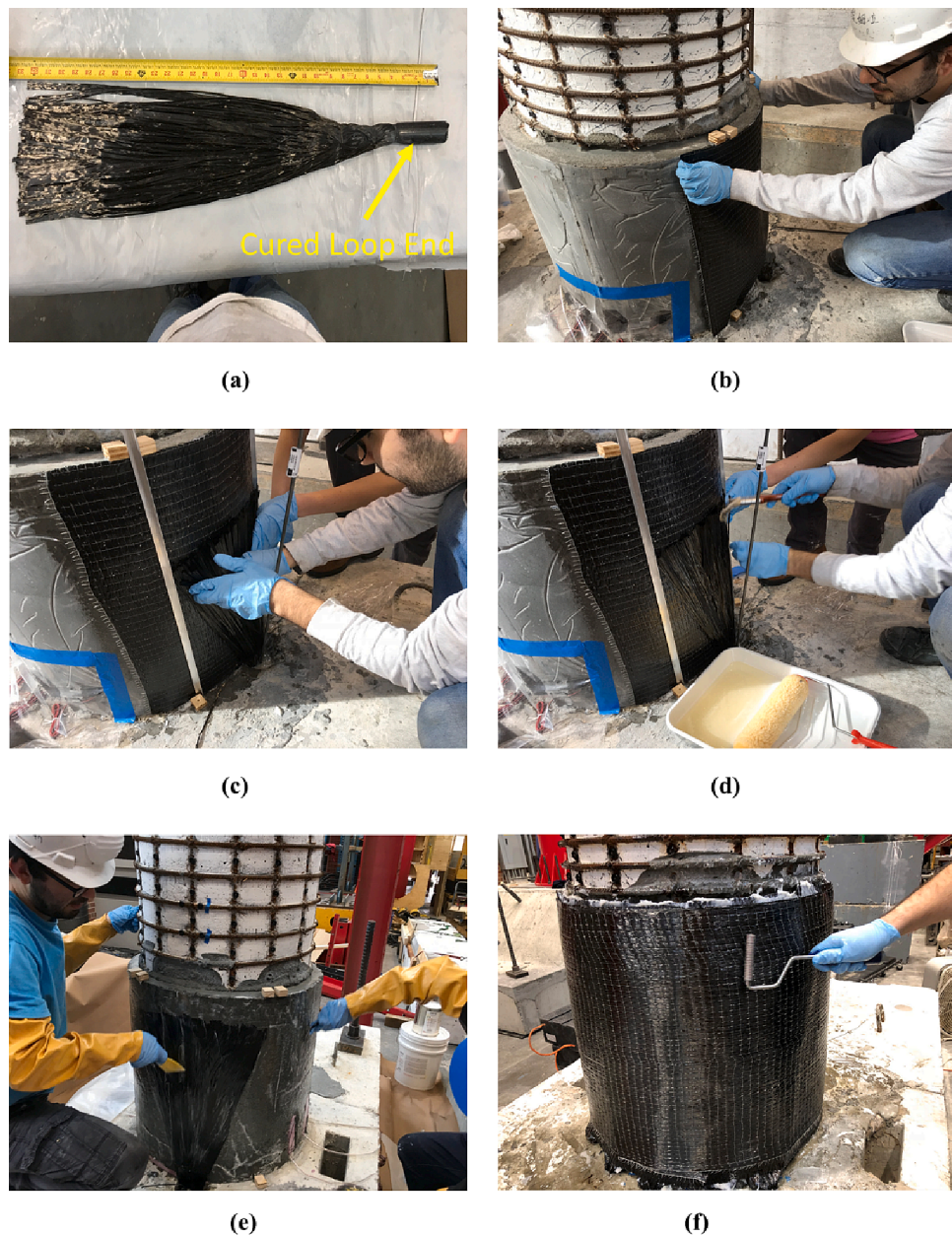
Fig. 18. CFRP Application a) Cured Loop End b) CFRP Laminate Application c) CF anchor Application and Splaying of Anchor Fan Fiber d) Anchor Fan Fiber Saturation e) Stretching Anchor Fan Fiber to Form Anchor Fan f) Transverse Wrap.
