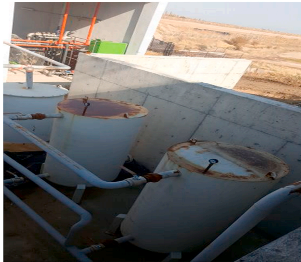
Fig. 4. Desulphurization unit and CHP connection line.
