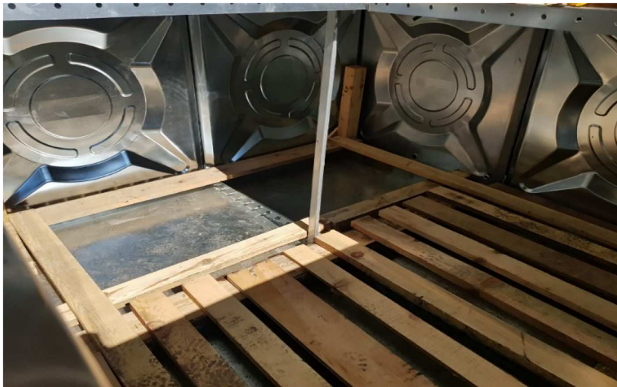
Figure 11. Construction of the platform where the wooden bases were placed in the pool.
