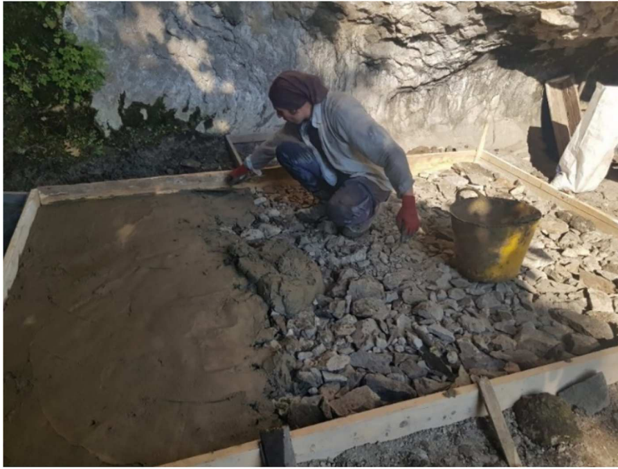
Figure 10. Construction of the flood basin on which the protection pool was positioned.
