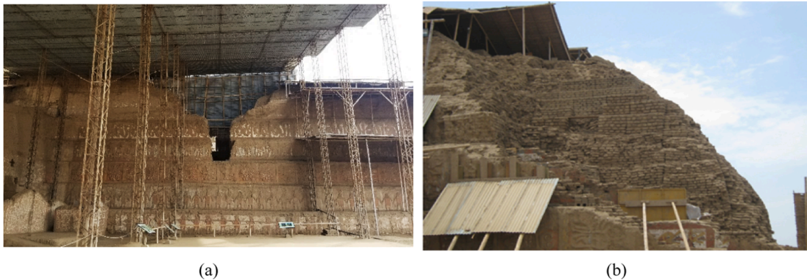
Fig. 5. Extant damage: (a) colonial “looter’s cut” on the North Façade and (b) collapse of the northwest corner.
