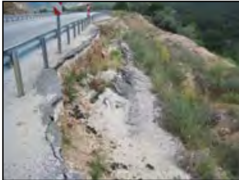
Figure 4. The Landslide and the deformations
