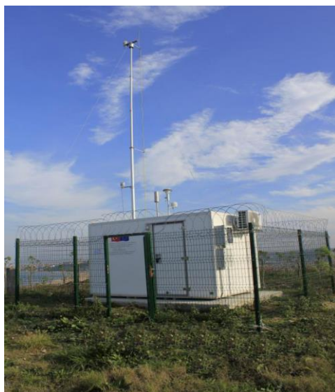
Figure 3. Kocaeli air quality monitoring station (central).
